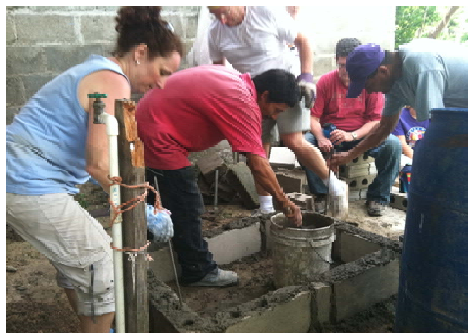
L to R: Elizabeth Sheehy, the author of this account, Bonifacio, Charlie Wilmott, Fr. Merrow and Fredy apply cement to the base of a new Pila.
