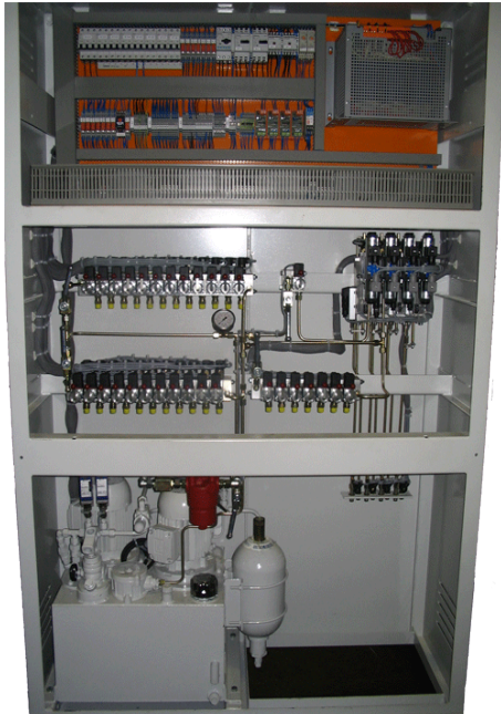
Inside solenoid valve cabinet
