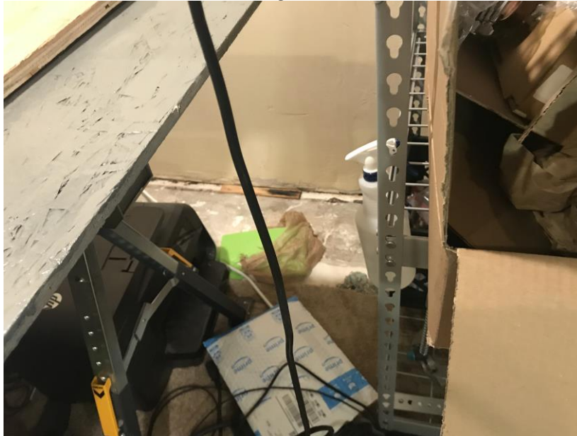
#5 rear corner leakage that occurred in 2019
