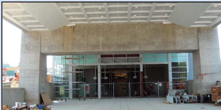
GROUND LEVEL ACCESS: Entrance gates will soon be installed at the ground level entrance along Tysons Boulevard to the Tysons Corner Metrorail Station. Photo by Stephen Barna, Dulles Corridor Metrorail Project
