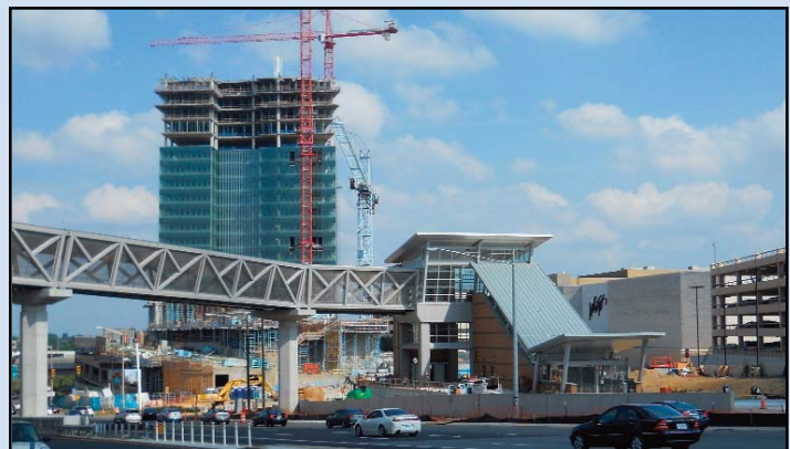
ACCESS COMPLETED: The pedestrian bridge and entrance pavilion at the Tysons Corner Metrorail Station are completed. In the background is construction of offices, a hotel and residential units by the owners of Tysons Corner Center, Macerich. Photo by Stephen Barna, Dulles Corridor Metrorail Project
