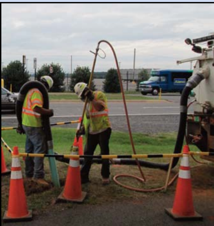
PHASE 2 UNDERWAY: Vacuum excavation for utility verification at proposed geotech boring location at the Dulles International Airport. Photo by Scott Evans, Dulles Corridor Metrorail Project
